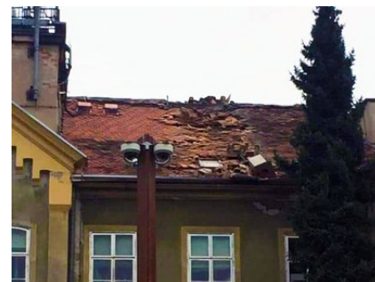
Earthquake damage outside. Some of the outside of the DHMZ building was also damaged.
